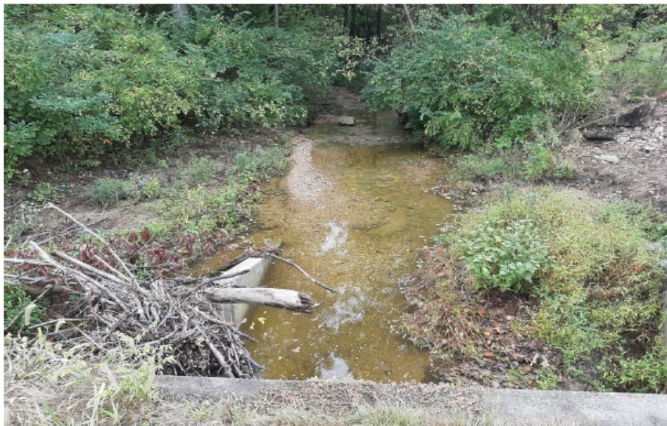
Photo 15. Upstream view of Tributary B from the culvert under Mexico Road, facing southwest.
