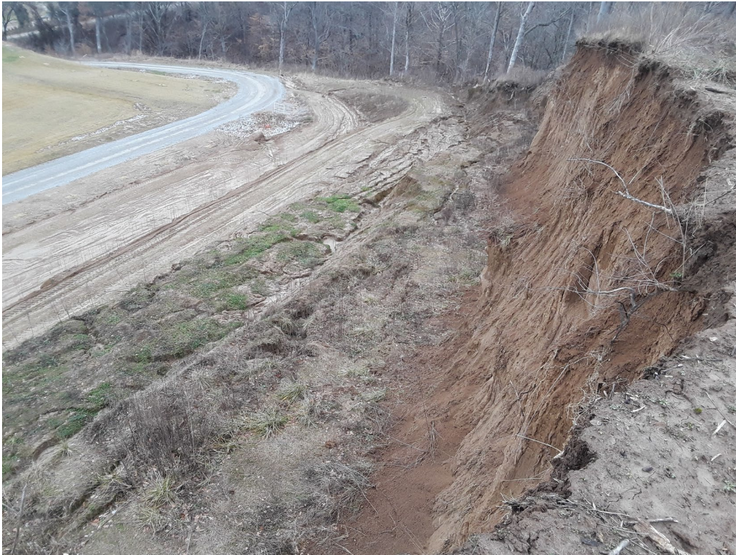
Figure 3. Existing terraced landscape that resulted from the 2017 borrow excavation. Best Management Practices were not fully implemented resulting in sparse vegetation and actively eroding soils on steep slopes. Picture was taken during a site visit on 18 January 2019.
