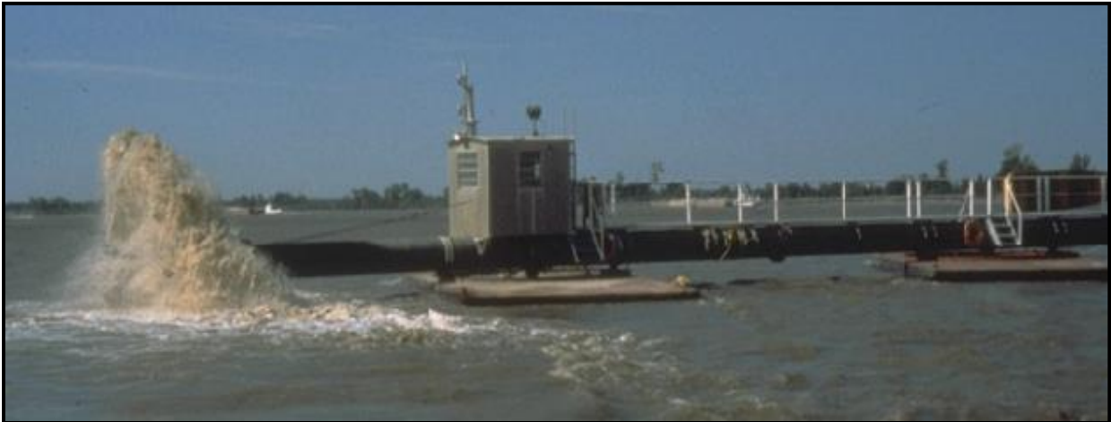
Photo 2. Example of rigid dredge pipe attached to pontoons.
