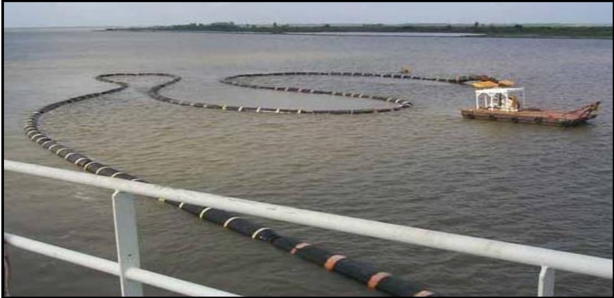
Photo 3. Example of flexible pipe.
