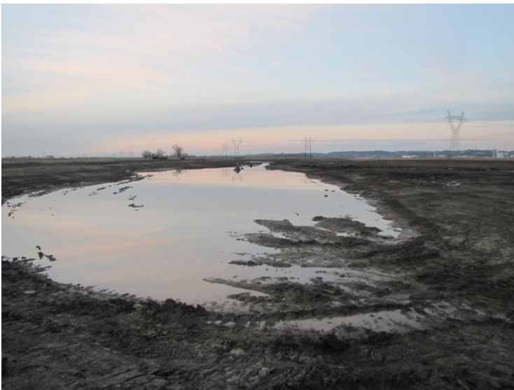
Photo 5. Example of an excavated swale with adjacent constructed ridges in West Alton, MO.
