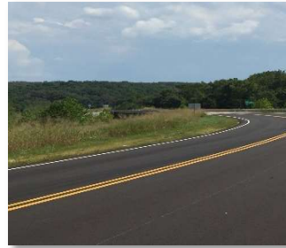
Final section of State Route D to be raised and relocated in partnership with MODOT.
