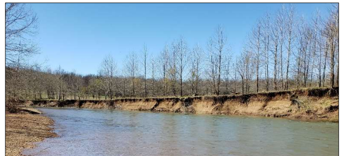
Unstable bank along the Big River that is contributing excessive sediment and heavy metals to the aquatic ecosystem
