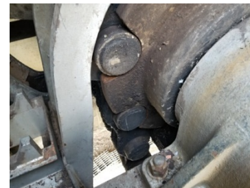
Lock 24 Dam Pier Rehab to include replacement of failing Gate Hoist Chains, Rehab of Bridge, and Repairs to Gates; $40M critical backlog, baseline awarded in FY20, task orders unfunded in FY21.
