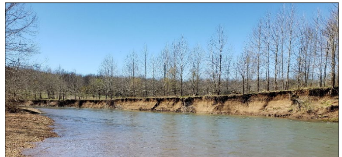
Unstable bank along Big River that is contributing excessive sediment and heavy metals to the aquatic ecosystem
