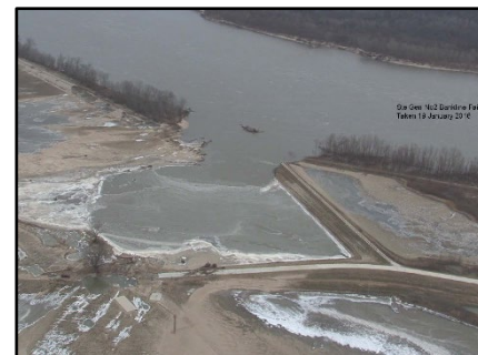
Bank-line failure at St. Genevieve, critical routine maintenance to revetments reduced in FY20, high risk of failures like this, with significant economic impact
