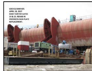
Lock 25 Dam Pier replacement of failing Gate Hoist Chains, Rehab of Bridge, and Repairs to Gate. $35M critical backlog executed in strategic task orders.
