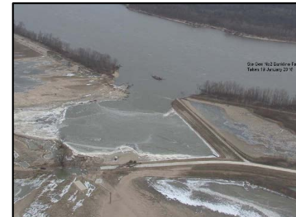
Bank-line failure at St. Genevieve, critical routine maintenance to revetments
