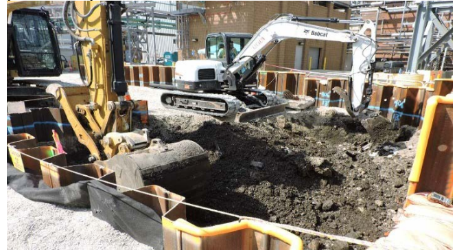
Excavation of contaminated soil at the Mallinckrodt Plant 1, former Building 17 area at St. Louis Downtown Site.
