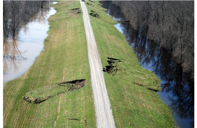
Typical Alton-Gale Levee Slides (2008 Flood)
