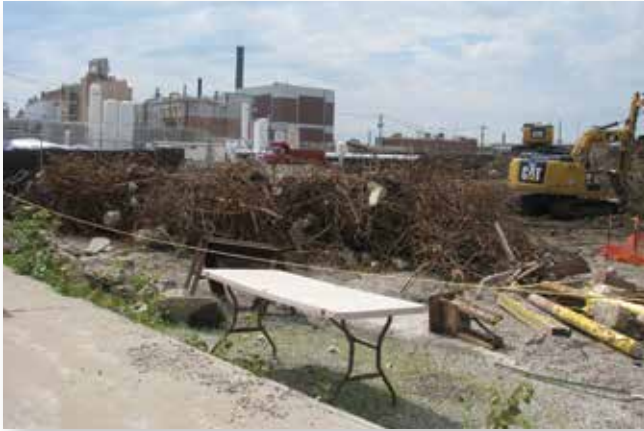
A portion of the former Building 101 footprint – St. Louis Downtown Site, including large amounts of rebar and metal that were separated, scanned and recycled.
