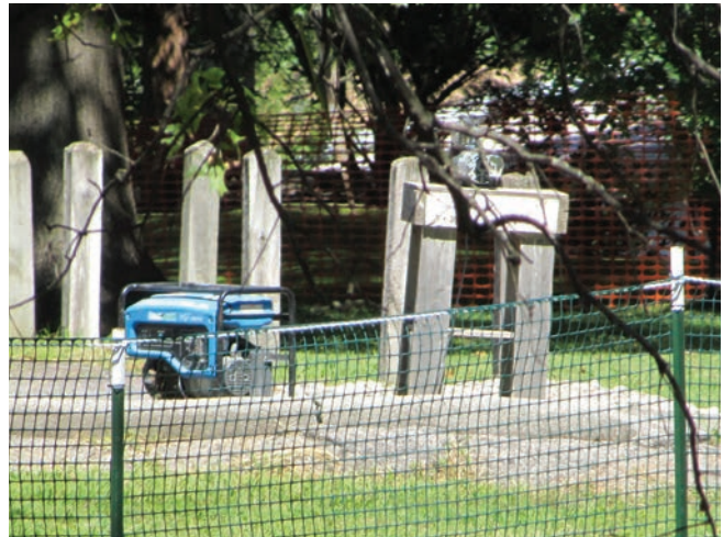
Inside an access-restricted FUSRAP work site, a generator on the left powers an air sampling unit on the right.
