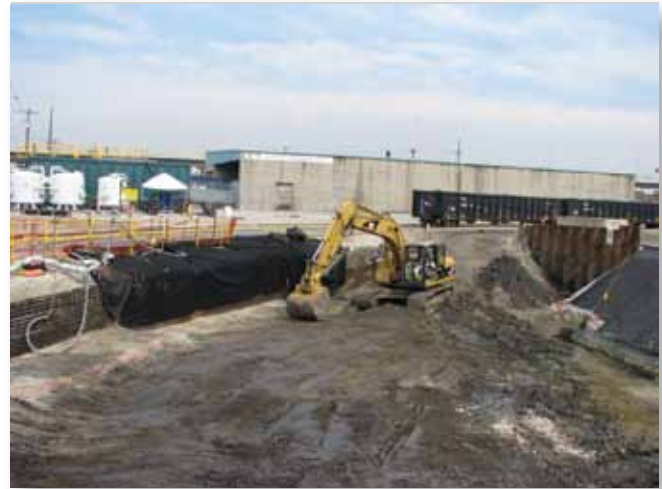
USACE has nearly remediated the sixth area in Plant 6WH, Phase 2 at the St. Louis Downtown Site.
