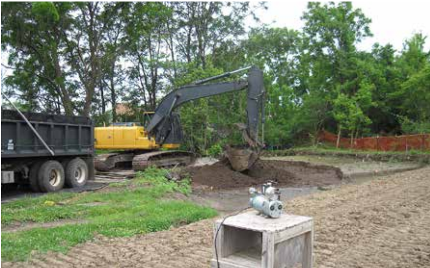
USACE completed remedial activities at Duchesne Park in February 2017. More than 8,600 cubic yards of contaminated material were removed. The City of Florissant has re-opened the restored park to the public.
