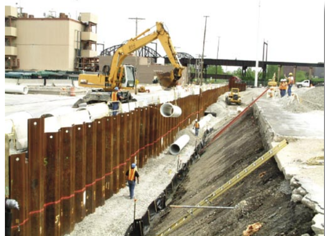
Sheet pile retaining wall preserves Destrehan Street stability during Plant 7N/7S remediation.
