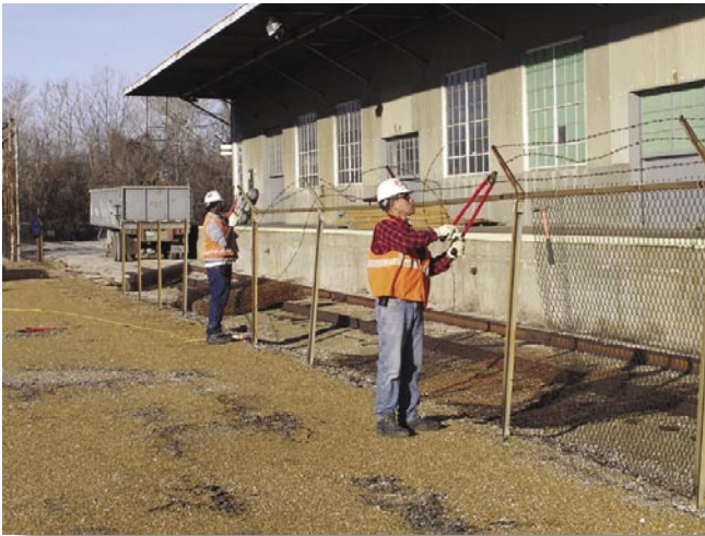
Laborers cut and remove fencing to allow equipment access to contaminated soil.
