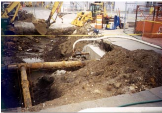
Workers cautiously excavate Plant 2 as they continue to encounter outdated utility lines.
