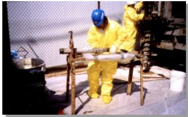
Systematically sampling Plants 1 and 6 will establish the excavation area and remediation volumes. The laborer shown here is working with a recently drilled soil sample.
