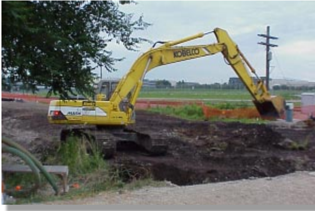
The East End removal action continued through the contractor turnover with the excavation of 5,200 cubic yards.
