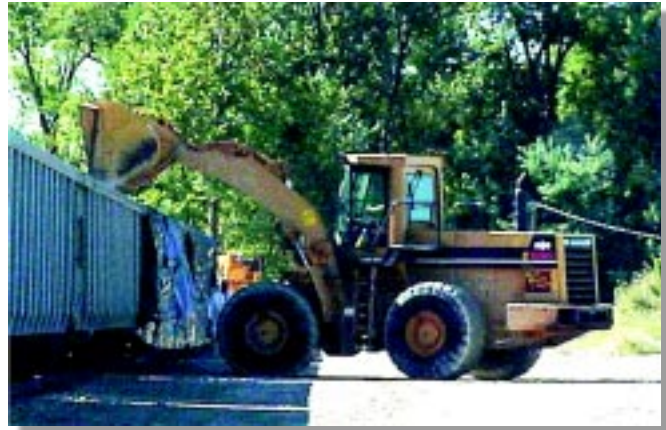
Removal of the final stockpile at HISS is nearly complete. Of the estimated 25,000 cubic yards comprising the Main Pile, roughly 20,200 cubic yards have been removed.
