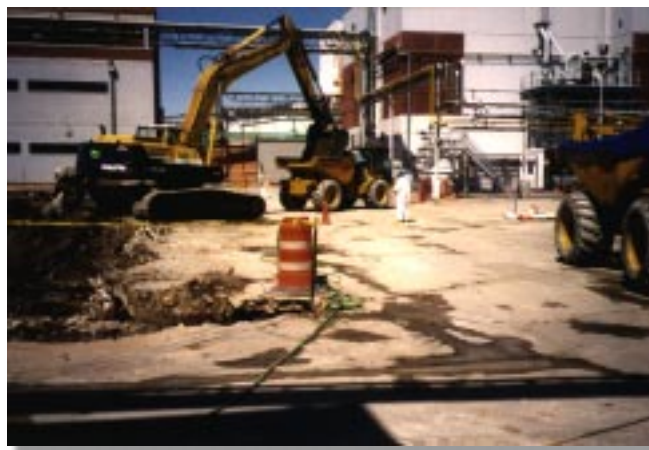
Excavators load material from the Plant 2 remediation work into trucks which transport the covered material to the SLDS railspur.
