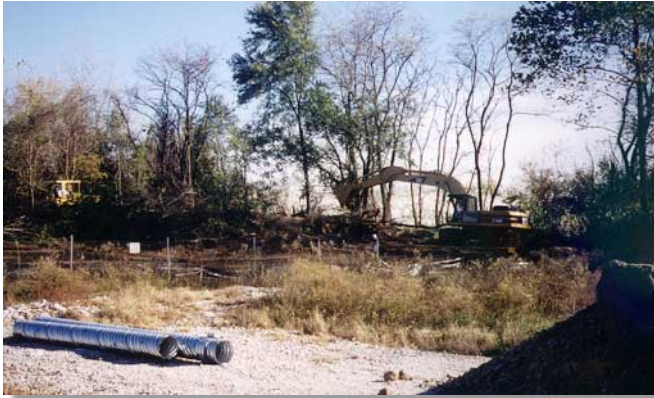
Crews begin clearing activities for the HISS railspur construction and sewerline encasement.
