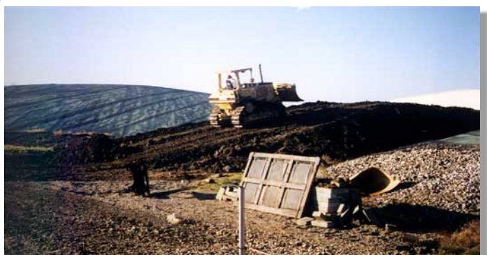
Construction crews grade soil for rail spur at the HISS site. Excess soil is temporarily stockpiled between the main and supplementary storage piles.
