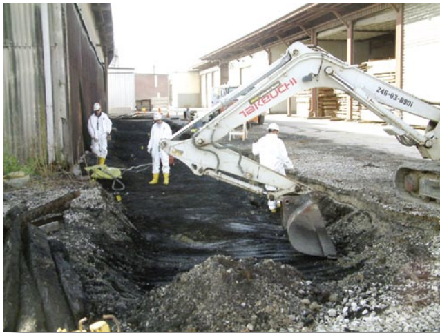
USACE started cleanup of the Thomas & Proetz property in November 2004 working in one small area at a time.
