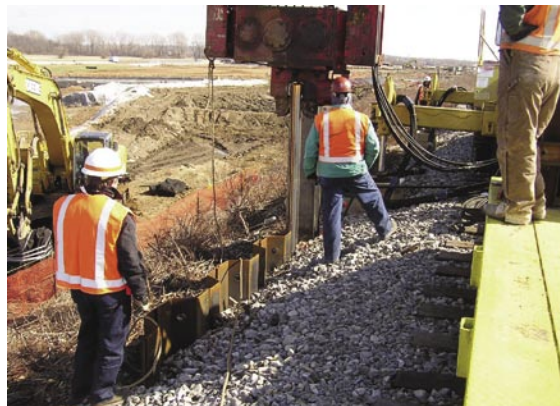
Crews are installing sheet piling along the Norfolk Southern Corporation rail line from a rail-mounted crane. Sheet piling is being installed to maintain the stability of the rail line during upcoming cleanup activities.
