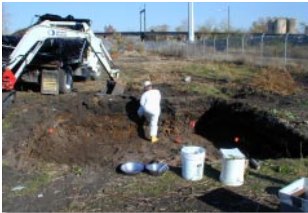
Remedial activities are well underway at the DT-7 vicinity property (located south of Mallinckrodt along Angelrodt Street).
