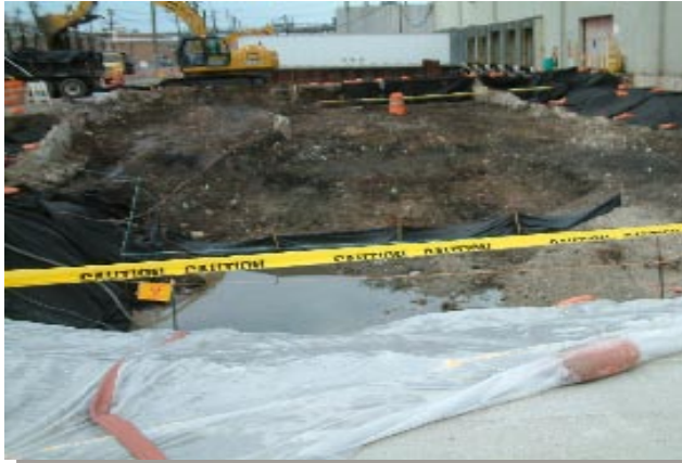
At the St. Louis Downtown Site (SLDS) crews had to deal with old concrete foundations, overhead and underground utilities and water infiltration during remediation of Plant 6W Half Phase I.
