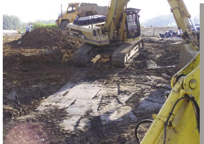
Removal activities in the Phase 4 and 5 work areas at the St. Louis Airport Site (SLAPS) are nearing completion.
