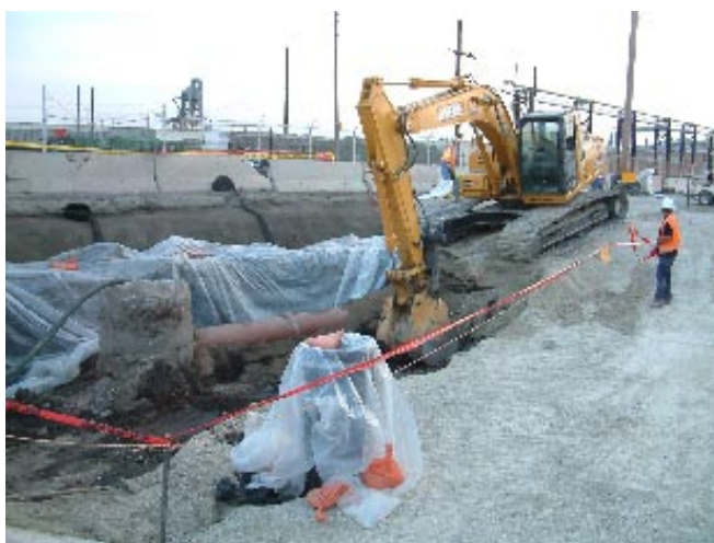
Remediation work continues at the southern boundary in Plant 6W Half Phase I Area 3.
