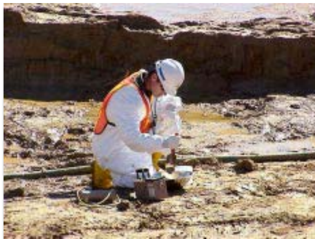
Removal activities are nearly finished in seven of the ten areas that make up the SLAPS East End Extension.
