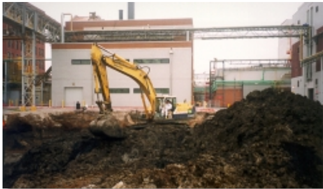
Excavation in Plant 2's main remediation area will continue once unexploded ordnance plans, which address the presence of the Civil War Ordnance, are approved.
