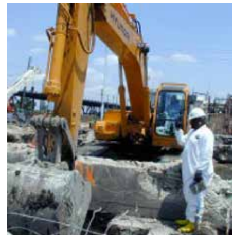
Crews removed thousands of cubic yards of soil and debris at the former Mallinckrodt buildings.
