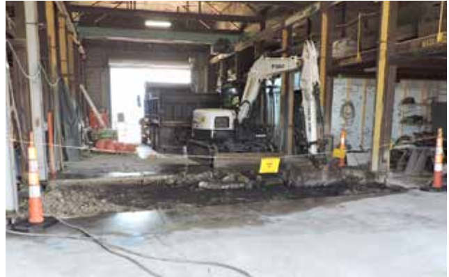
Remedial activities at the Heintz Steel property on the St. Louis Downtown Site.
