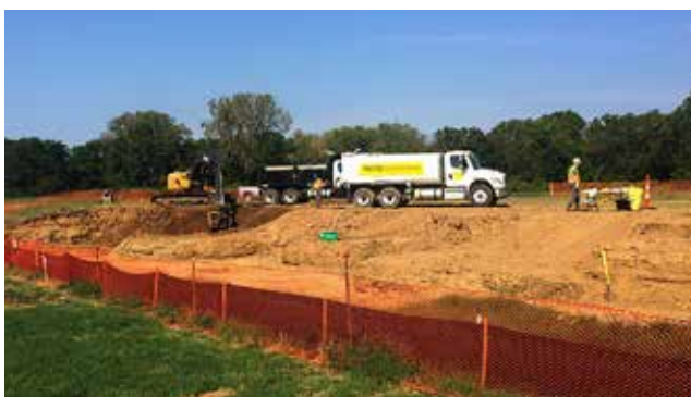
Contractors perform remedial activities at Ballfields Phase 2B across McDonnell Boulevard from the St. Louis Airport Site (SLAPS).
