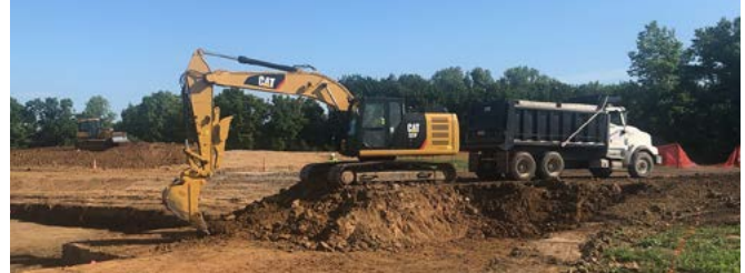
The contractor removes low-level radioactive material from Area 1 of the former Ballfields Phase 2B in North St. Louis County with a track-mounted excavator Wednesday, July 18, 2018.
