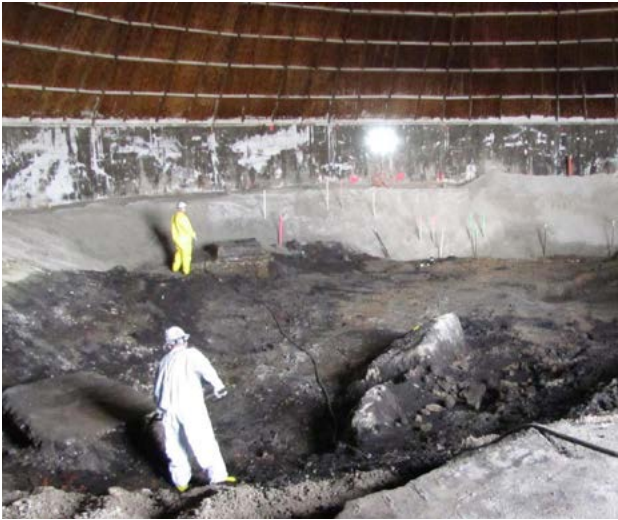
Contractors perform remedial activities at the Gunther Salt Property on the St. Louis Downtown Site (SLDS) Monday, April 8, 2019.
