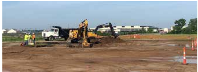
After finishing discharging water through a micron filter, the crew prepares to begin the remedial excavation and hauling of contaminated material from the Ballfields Phase 2B project to the load-out facility Tuesday, May 22, 2018.
