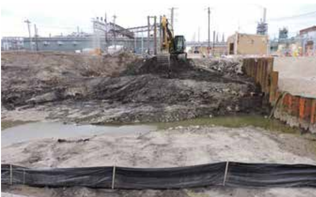
An excavator operator from contractor HydroGeoLogic Inc. (HGL) performs remediation at Destrehan Street at the St. Louis Downtown Site (SLDS) Wednesday, April 18, 2018.
