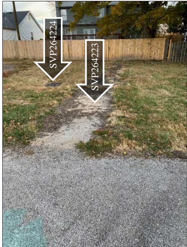
Image 2. Pavement Sediment Northeast of Basketball Courts
