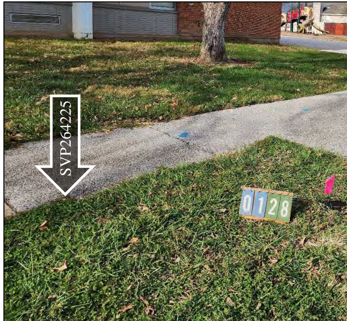
Image 3. Pavement Sediment Southwest of Basketball Courts
