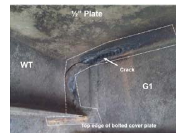
Critical cracking in upstream vertical liftgate at Mel Price Locks and Dam, 2 lengthy unscheduled closures
