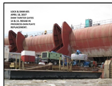
Lock and Dam 25 Dam Pier Rehab Contract (before/after) includes replacement of Failing Tainter Gate Hoisting Chains and Sprockets, Rehab of Service Bridge and Repairs to Tainter Gate Structures. Total of $35M critical backlog work executed in strategically planned task orders.
