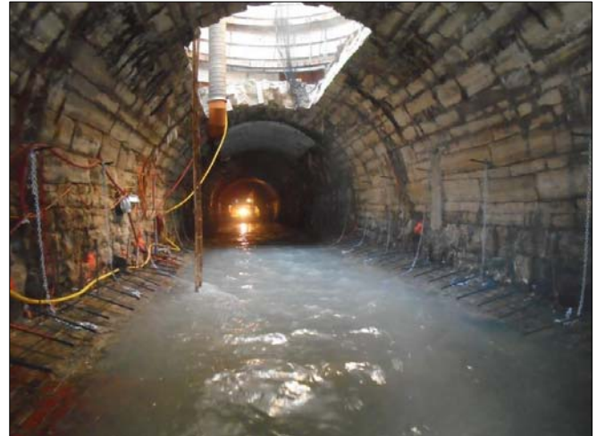
Old Mill Creek Sewer Line Prior to Repairs
