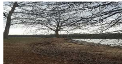
Recreation area shoreline damage due to flooding
