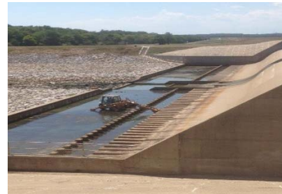
Stilling Basin in need of repairs
