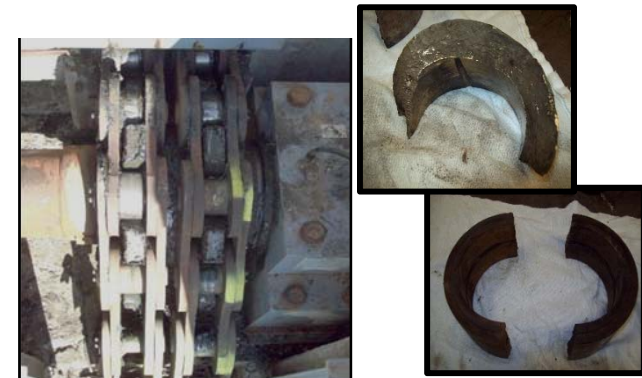
Failed Liftgate Hoisting Rollers at Locks 27
