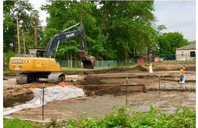
Remediation at Palm Drive Properties along Coldwater Creek was completed July 2017; Ballfields Phase 2B site along Coldwater Creek was initiated in August 2017.
