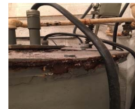
One of the corroded lift station in the power plant
