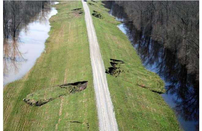
Typical Alton-Gale Levee Slides (2008 Flood)
