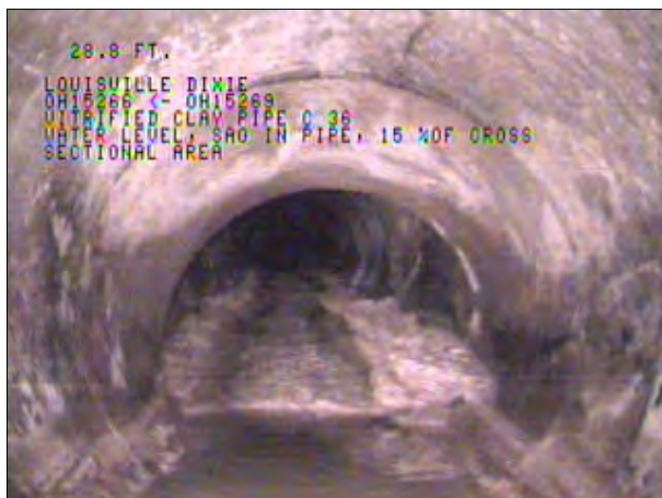
Photo: OH15269_OH15266124455_05112009_A.JPG, VCR No.: FLOOD WALL#2, 01:43:58 28.8FT, Water Level, Sag in pipe, 15 %of cross sectional area
