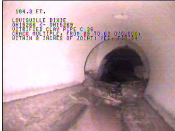
Photo: OH15269_OH15266124848_05112009_A.JPG, VCR No.: FLOOD WALL#2, 01:46:48 104.3FT, Crack Multiple, from 09 to 03 o'clock, within 8 inches of joint: YES, Finish
