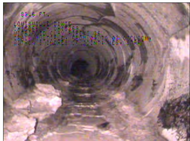
Photo: OH15269_OH15266124807_05112009_A.JPG, VCR No.: FLOOD WALL#2, 01:46:12 83.6FT, Crack Multiple, from 09 to 03 o'clock, within 8 inches of joint: YES, Start
