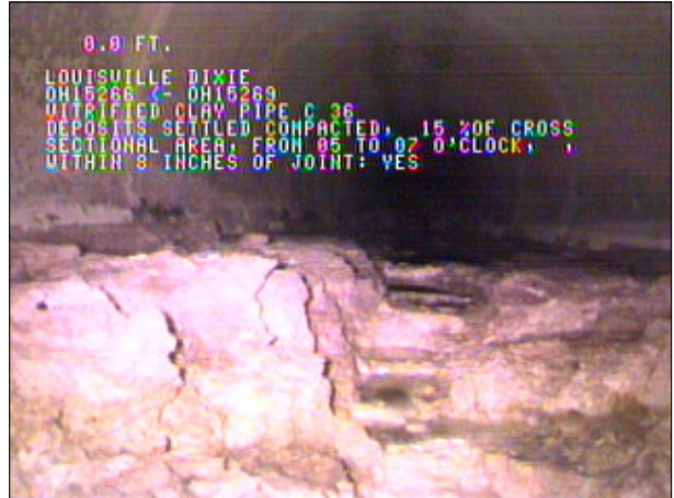
Photo: OH15269_OH15266124326_05112009_A.JPG, VCR No.: FLOOD WALL#2, 01:42:36 0FT, Deposits Settled Compacted, 15 %of cross sectional area, from 05 to 07 o'clock, , within 8 inches of joint: YES
