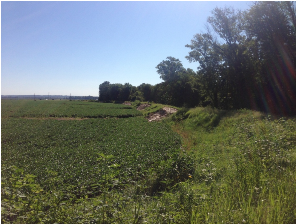
Figure 3. Creek-side scour and multiple breach locations.
