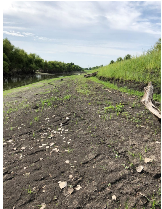
Figure 2. Embankment slide along the unprotected side of the Elm Point levee.
