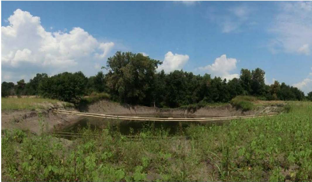
Figure 3. Breach on Chouteau Island Levee.
