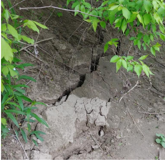
Figure 4. Stress cracks present on the bank slope
