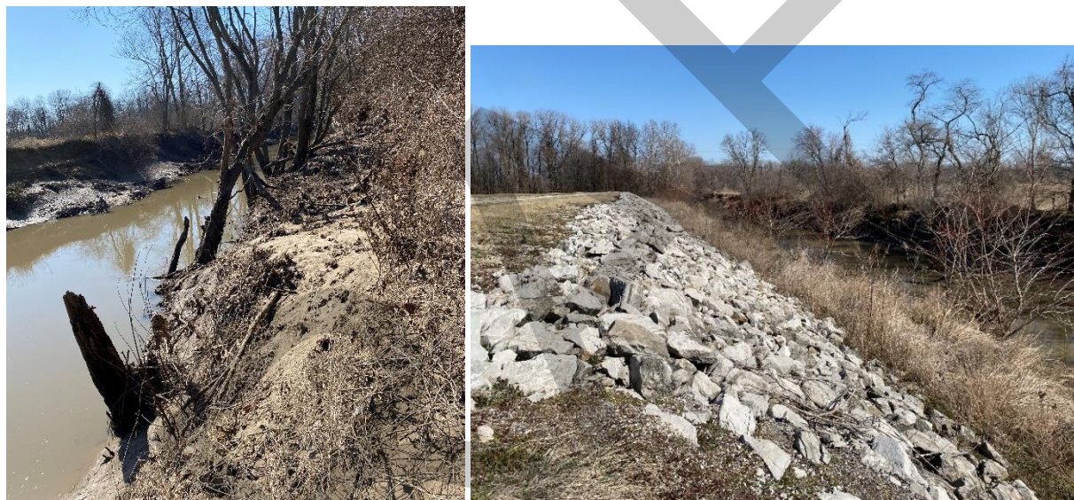
Figure 5. Comparison of existing streambank conditions (left) to completed 2002 stone revetment project (right) immediately adjacent to potential project location on Silver Creek.
