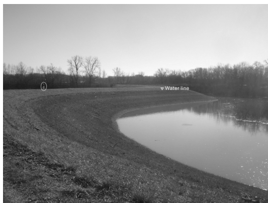
Figure 5. The Valley Park levee looking south, only 1 hour after the flood gates were reopened on January 2, 2016. The floodwater level (dark) almost breached the levee and exceeded the estimated level for a “100-year flood” (FEMA, 1995) by nearly 2 m, forcing evacuation of the protected area to the left. Bicyclist (circled) on levee top shows scale. Photo by Robert E. Criss.
