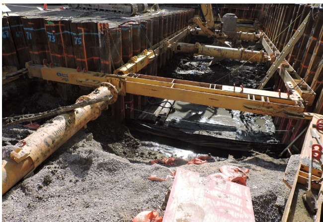
The FUSRAP team uses an excavator to remove contaminated soil within the shored portion of the St. Louis Downtown Site's Plant 1 Former Building 17 area Tuesday, Oct. 24, 2017.
